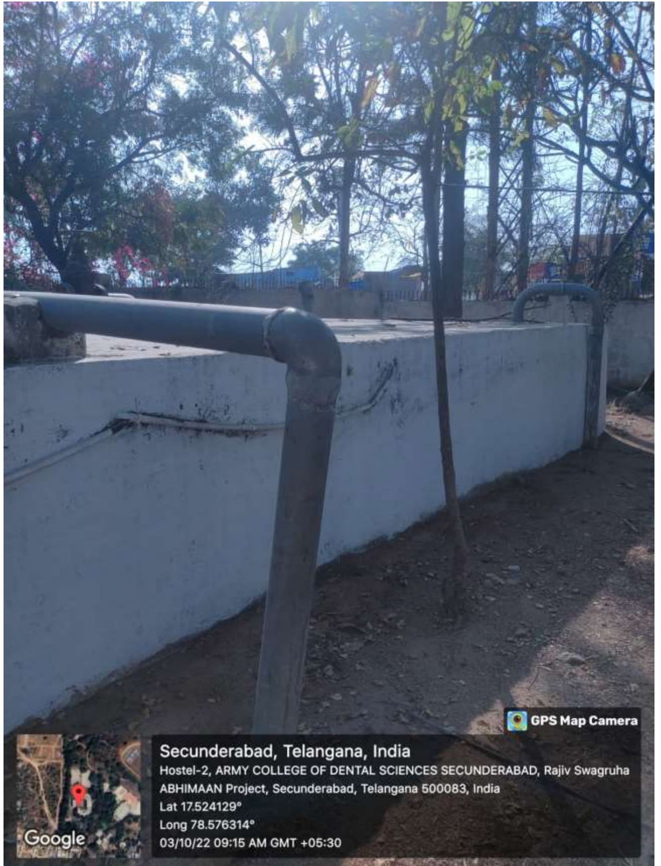
Fig- 19: Water pipeline distribution outside college
