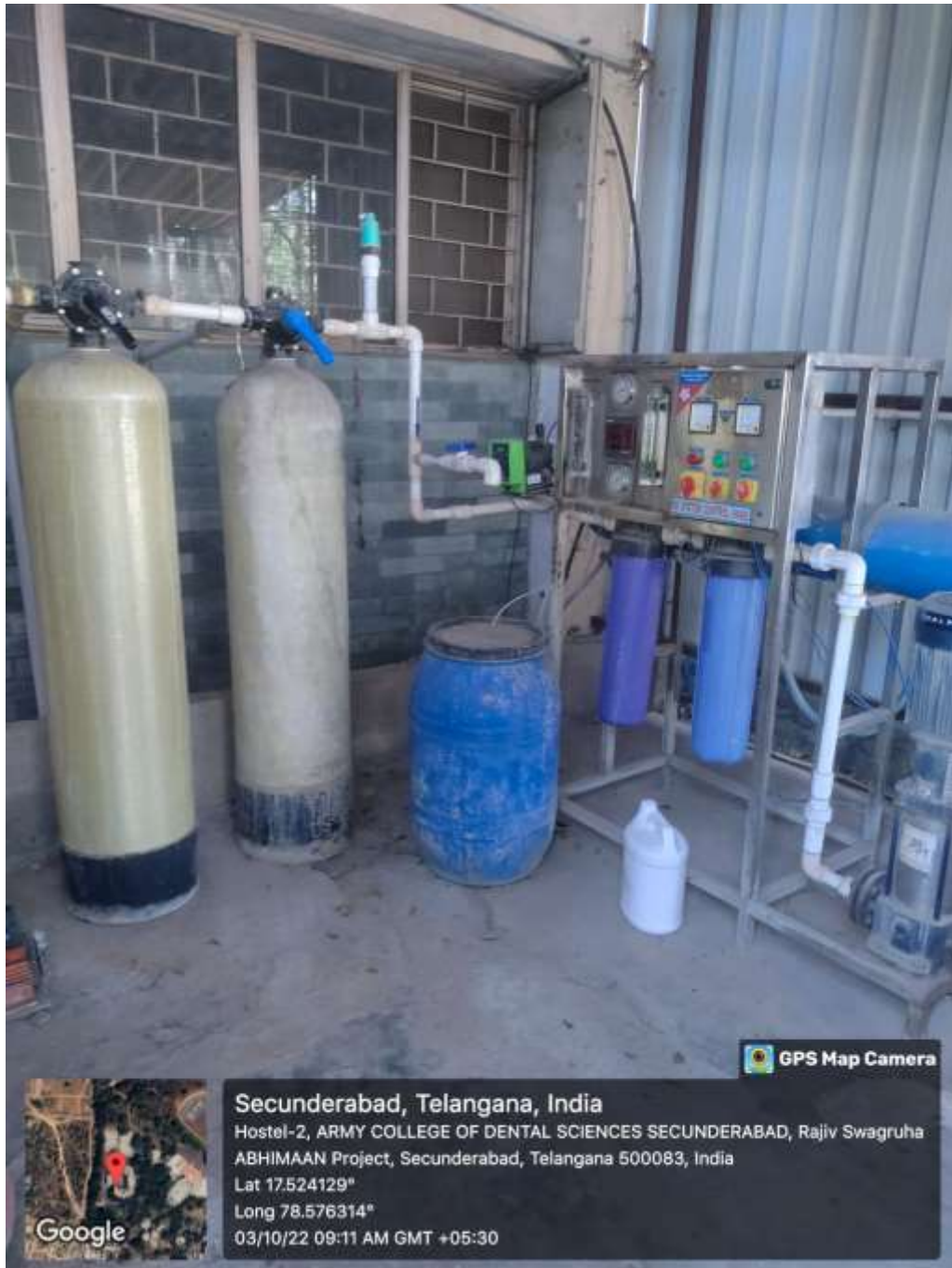
Fig-18: RO water plant in college campus
