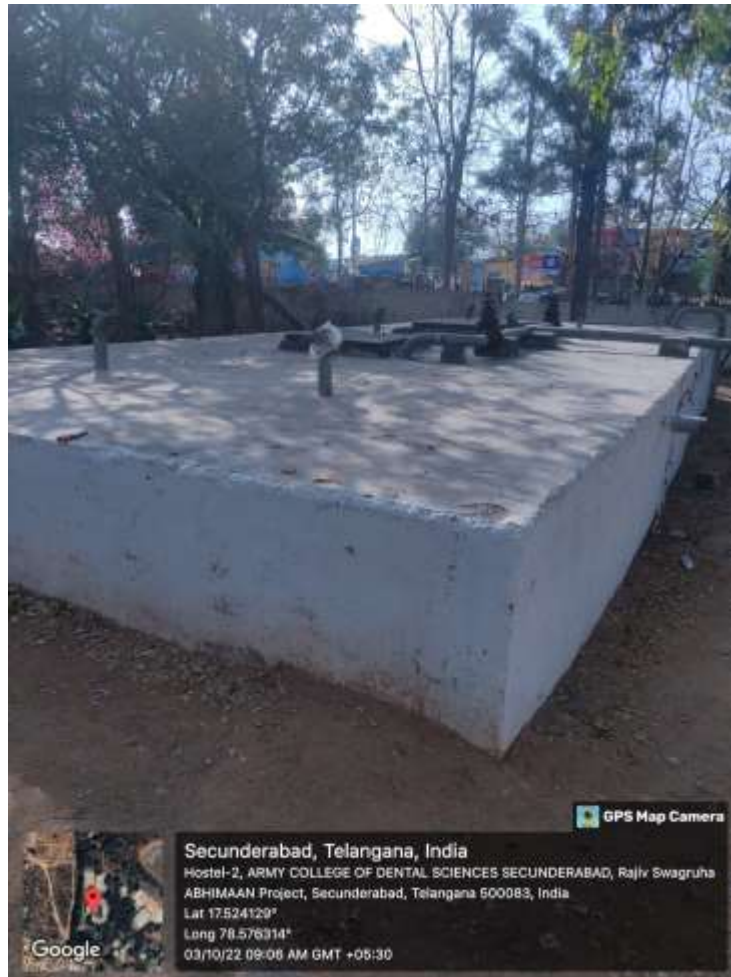
Fig-7: Water tank in the college premises
