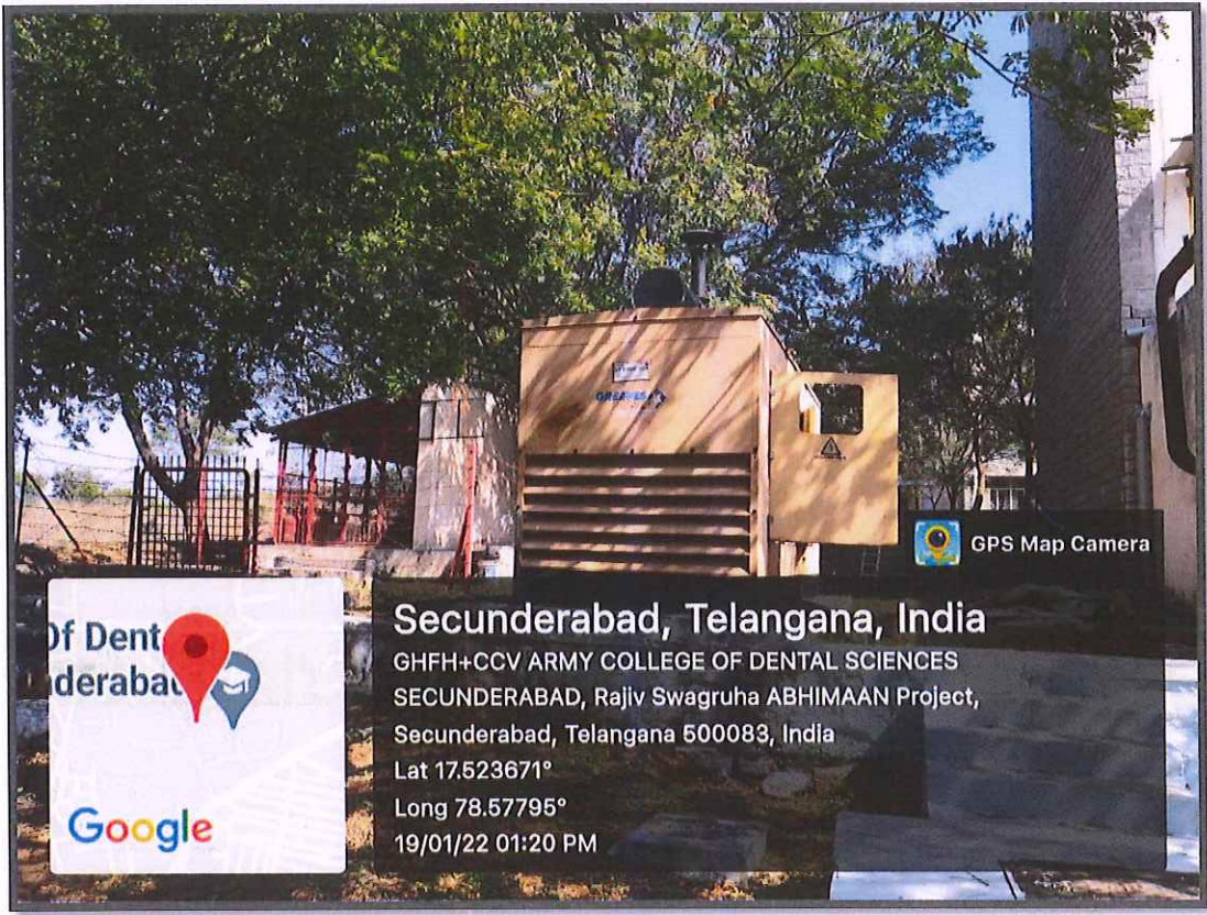
Fig-15: 250 KV capacity Generator in college campus
