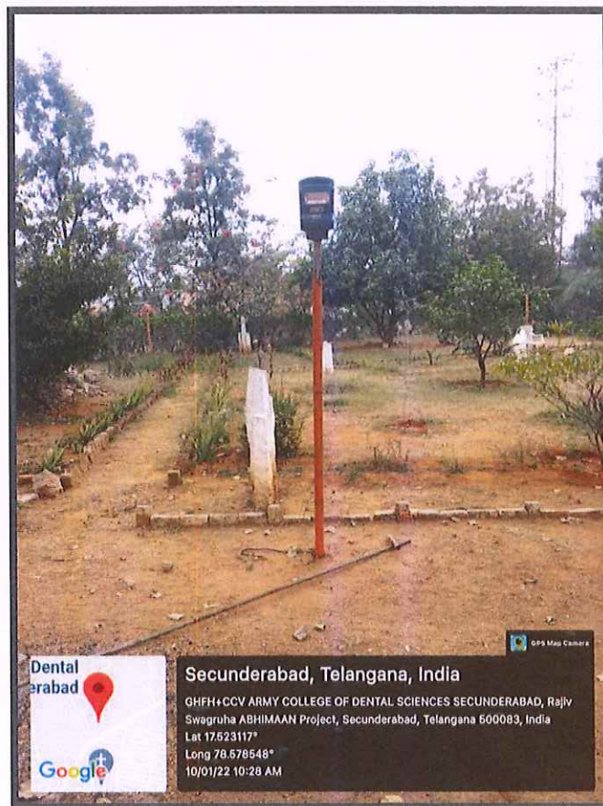
Fig-6: Solar flood light installed in college garden
