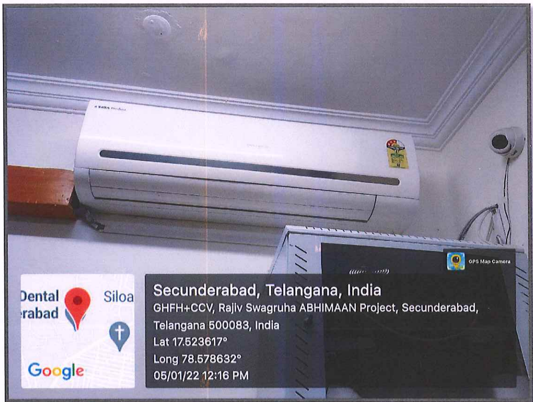
Fig-19: 3-star Air conditioner unit installed in various departments
