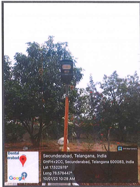
Fig-5: Solar flood light installed in the college garden
