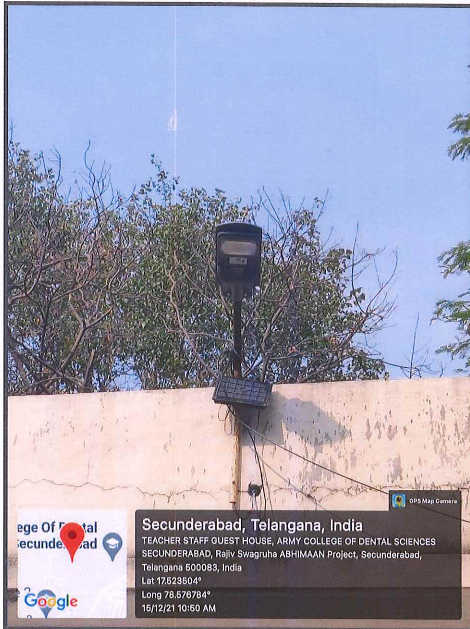
Fig-4: Solar flood light installed at staff quarters parking area
