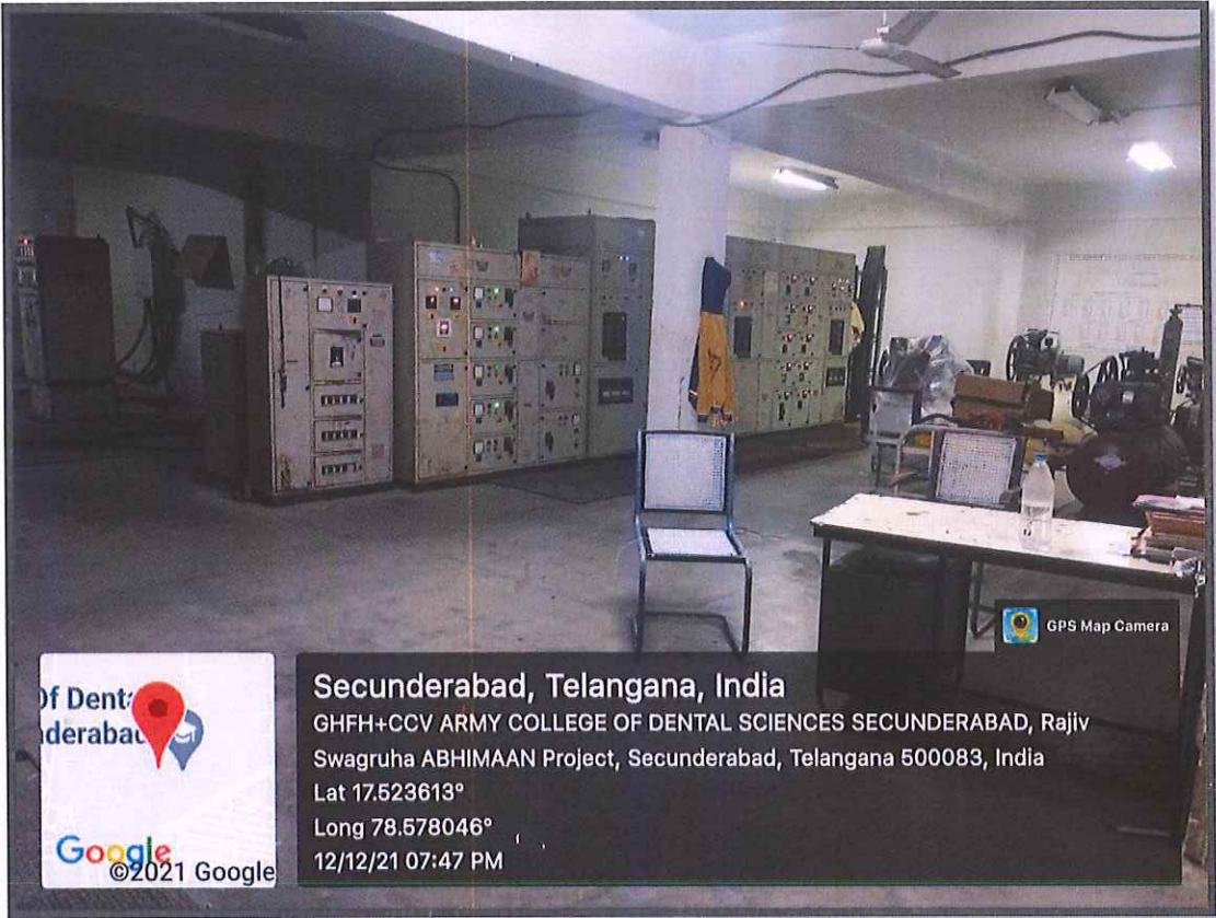
Fig-14: Generator room in college campus
