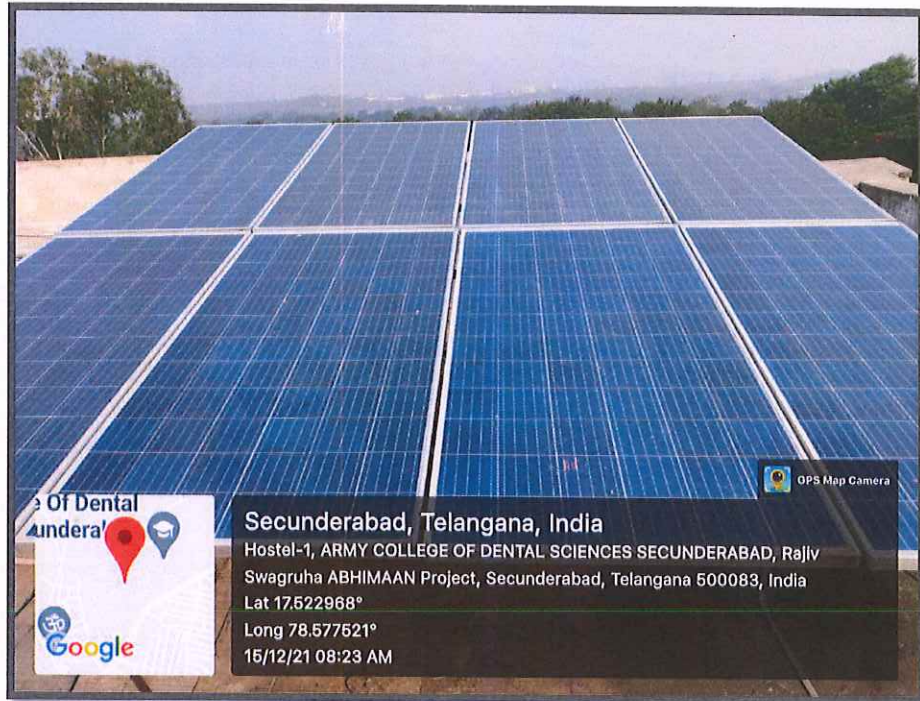
Fig-1: 25 KW solar roof top power grid
