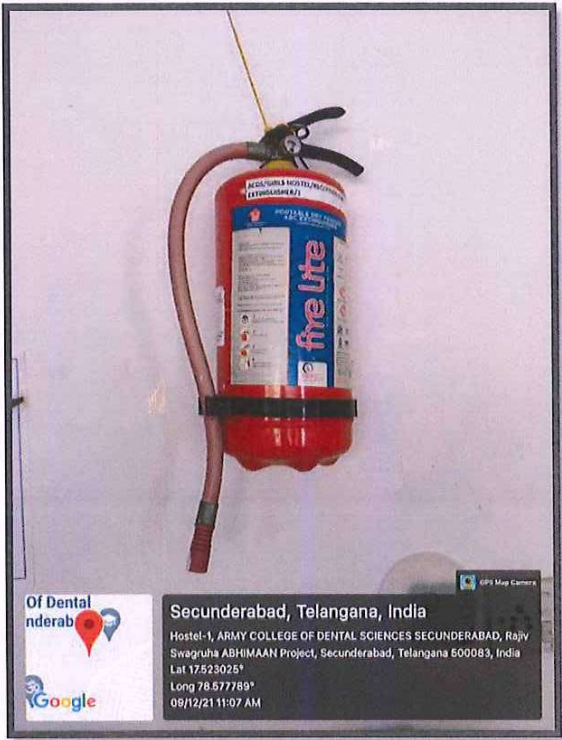
Fig-21: Fire safety equipment in Boy's hostel
